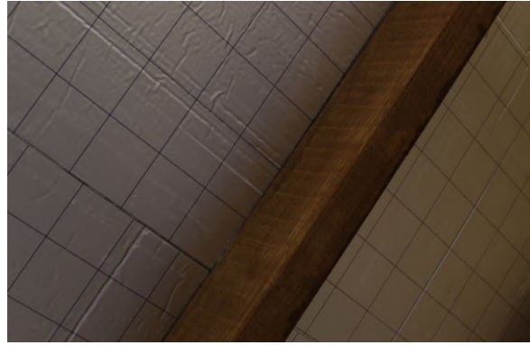
Photo 05 Roof view from inside without full boarding This requires finishing with, for example, dry plaster.
