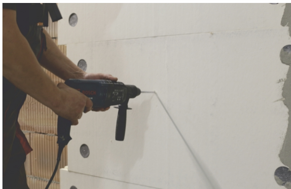
STAGE IV a) Drilling a hole in the wall for an anchor screw sleeve
