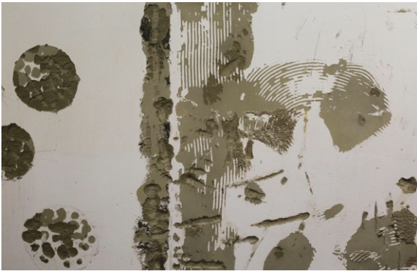
Figure 1. Cavities to be filled with adhesive
