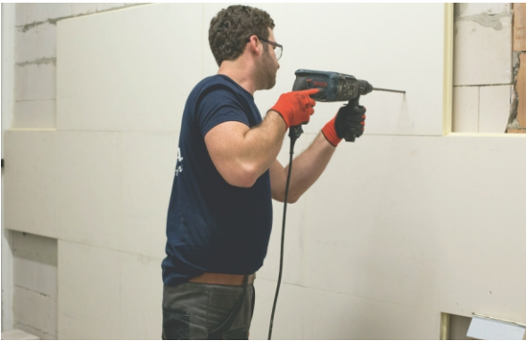
STAGE IV a) Drilling a hole in the wall for an anchor screw sleeve
